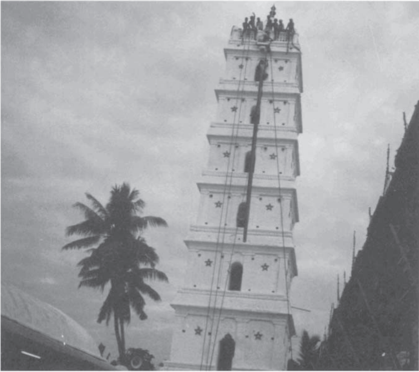
Plate 3.2 The erection of the flagpoles on one of the five minarets, built by the Maratha ruler Pratap Simha, Tanjavur, Tamil Nadu
